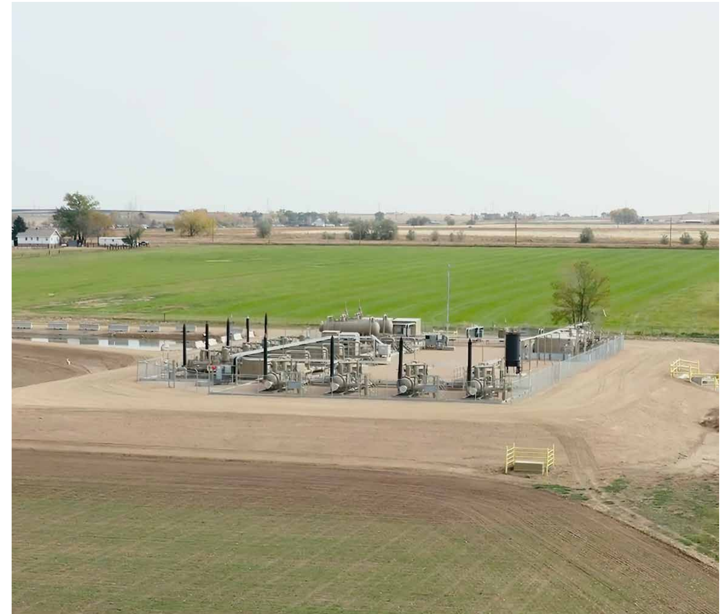
Tankless Facility Design
